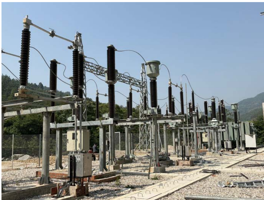
Figure: API Tower at Powerhouse Switchyards
