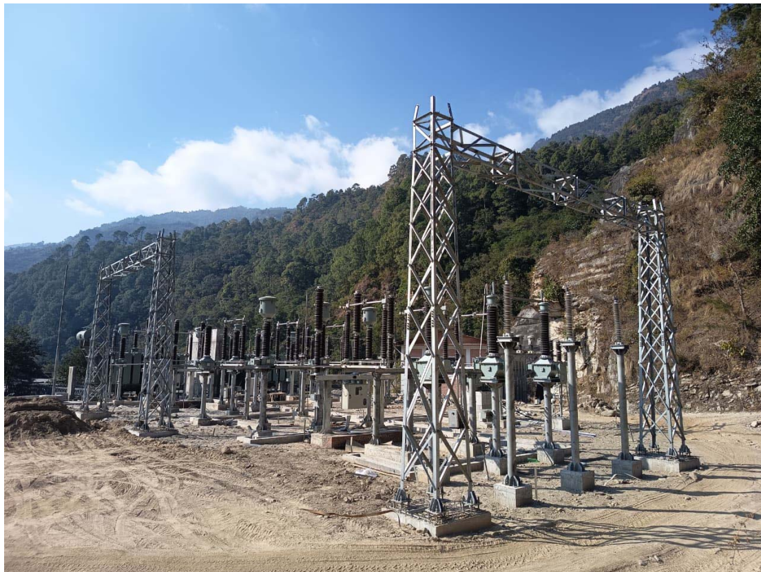
Switchyard area of the power
