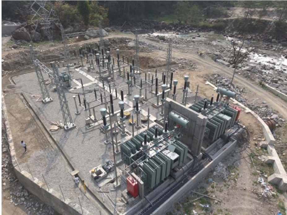
Figure: Power House Switchward
